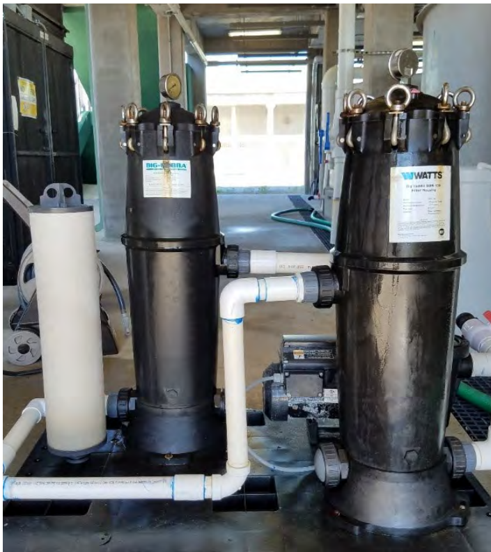
FIGURE 2. Filtration equipment installed on a pallet with quick disconnect and union fittings at the Louisiana Sea Grant Oyster Research Hatchery in Grand Isle, Louisiana. Photo courtesy of John Supan
