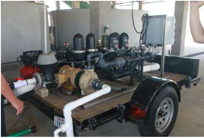
FIGURE 1. Filtration equipment installed on a trailer with quick disconnect and union fittings at the Louisiana Sea Grant Oyster Research Hatchery in Grand Isle, Louisiana. Photo courtesy of University of Florida/IFAS Shellfish Extension
